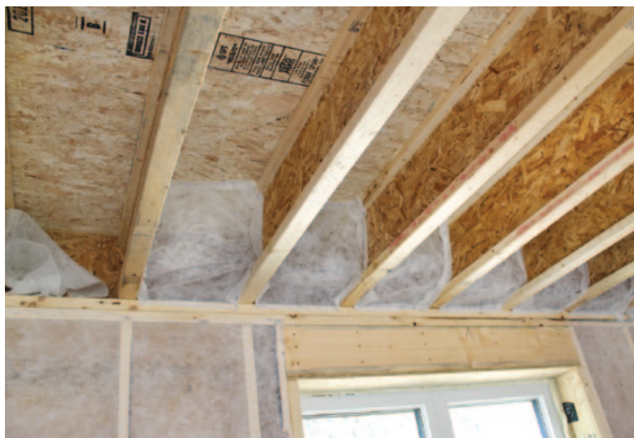
Figure 7. A strip of netting between a top-plate nailer and the facing joist makes it possible to dense-pack this area of the band joist (top). Netting stapled between the joist ends is filled with cellulose to form insulating and air-sealing "pillows" (above).
